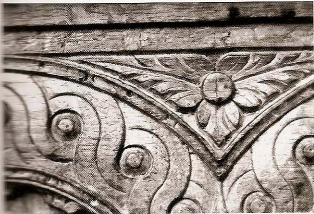
Fig 1.3 Panelwork at Abbey Dore Church which has been vigorously executed with a few simple tools
