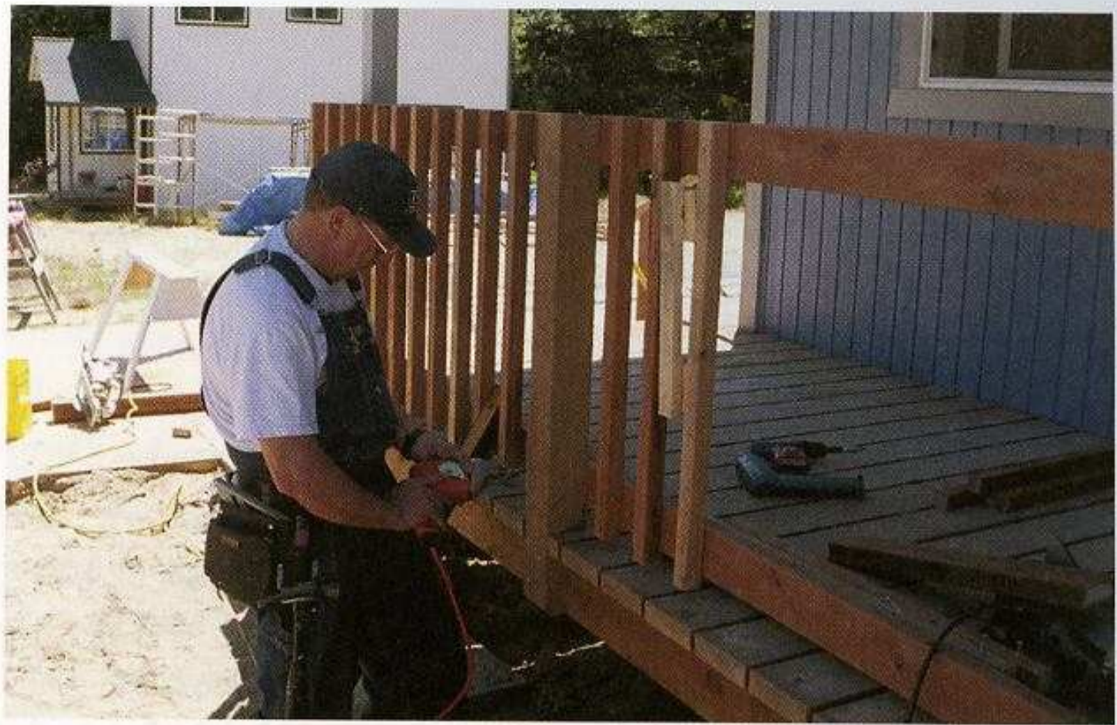
POSTS, RAILS, AND BALUSTERS MUST BE PRECISE. The clean lines on a finished porch or deck depend on accurate railing installation. Here, the posts are notched to fit against the rim joist. The ends of the decking boards overhang beyond the rim joist, even with posts.
