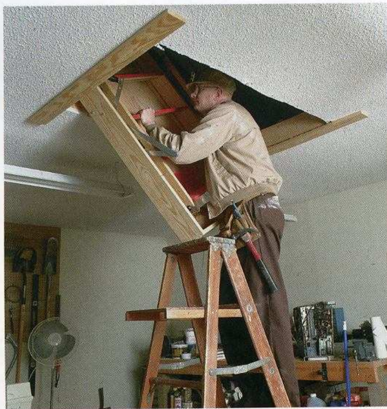
TEMPORARY LEDGERS SIMPLIFY INSTALLATION. A pair of boards can be screwed to ceiling framing, supporting the ends of the drop-down staircase until it's secured. [Photo by Jefferson Kolle, courtesy Fine Homebuilding magazine, © The Taunton Press, Inc.]
