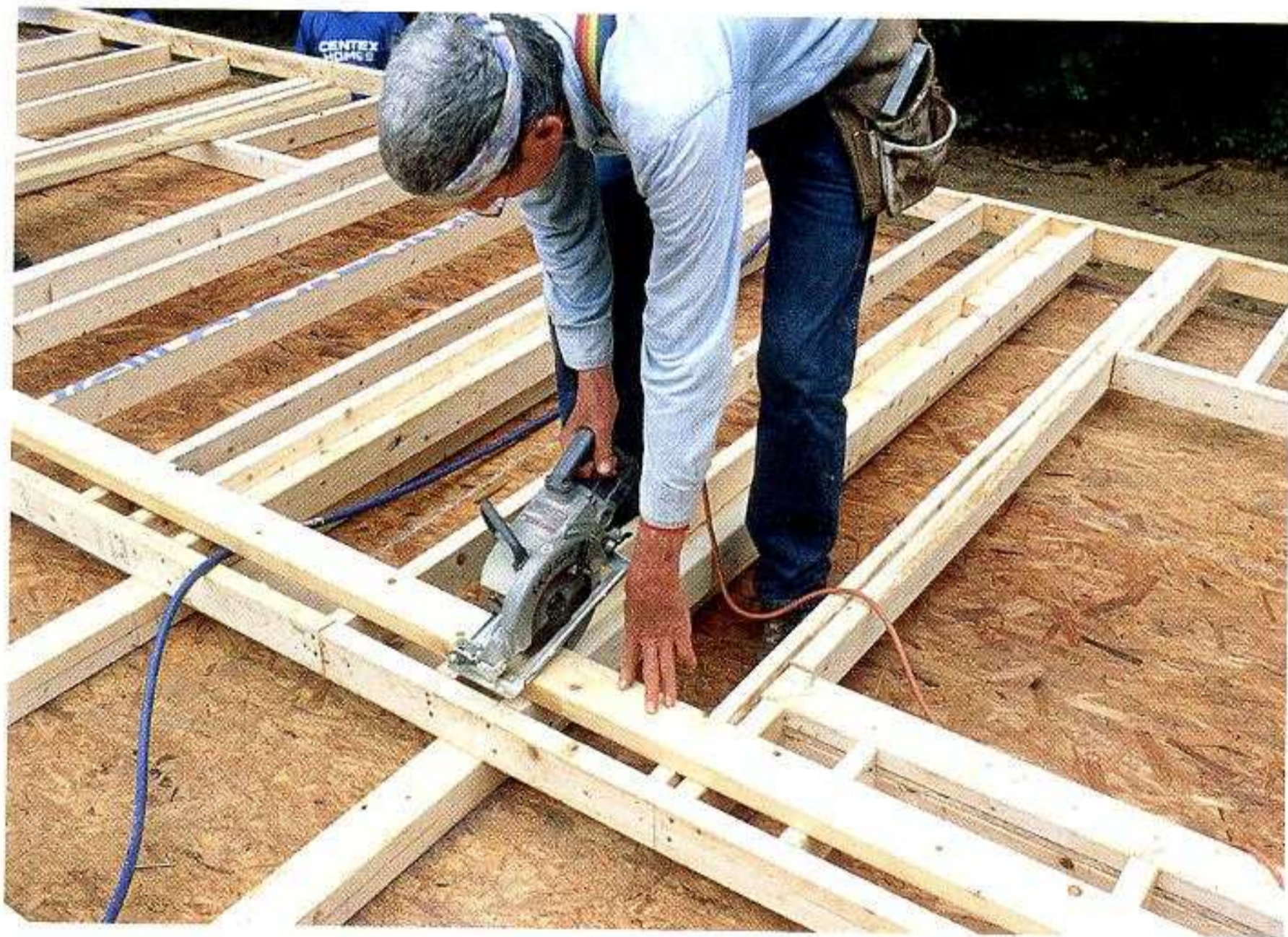
CUT THE DOUBLE TOP PLATE. With the bottom plate nailed off, cut the double top plate in place, following the layout marks on the top plate.
