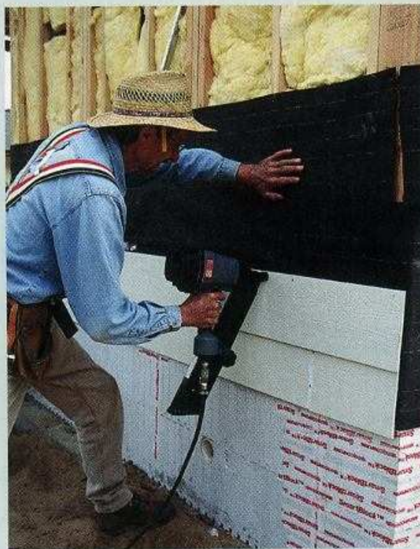
INSTALLING THE SIDING. Fiber-cement panels can be installed over exterior sheathing or nailed against housewrap or felt fastened to the framing.
