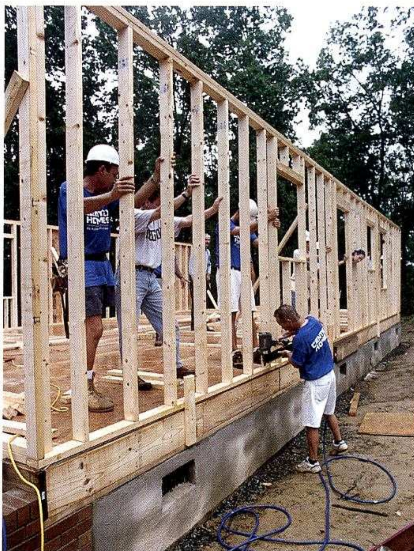
NAIL THE BOTTOM PLATE. One worker nails while others steady the wall. The short 2x4s nailed to the rim joist prevent the bottom plate from sliding off the floor when the wall is raised.
