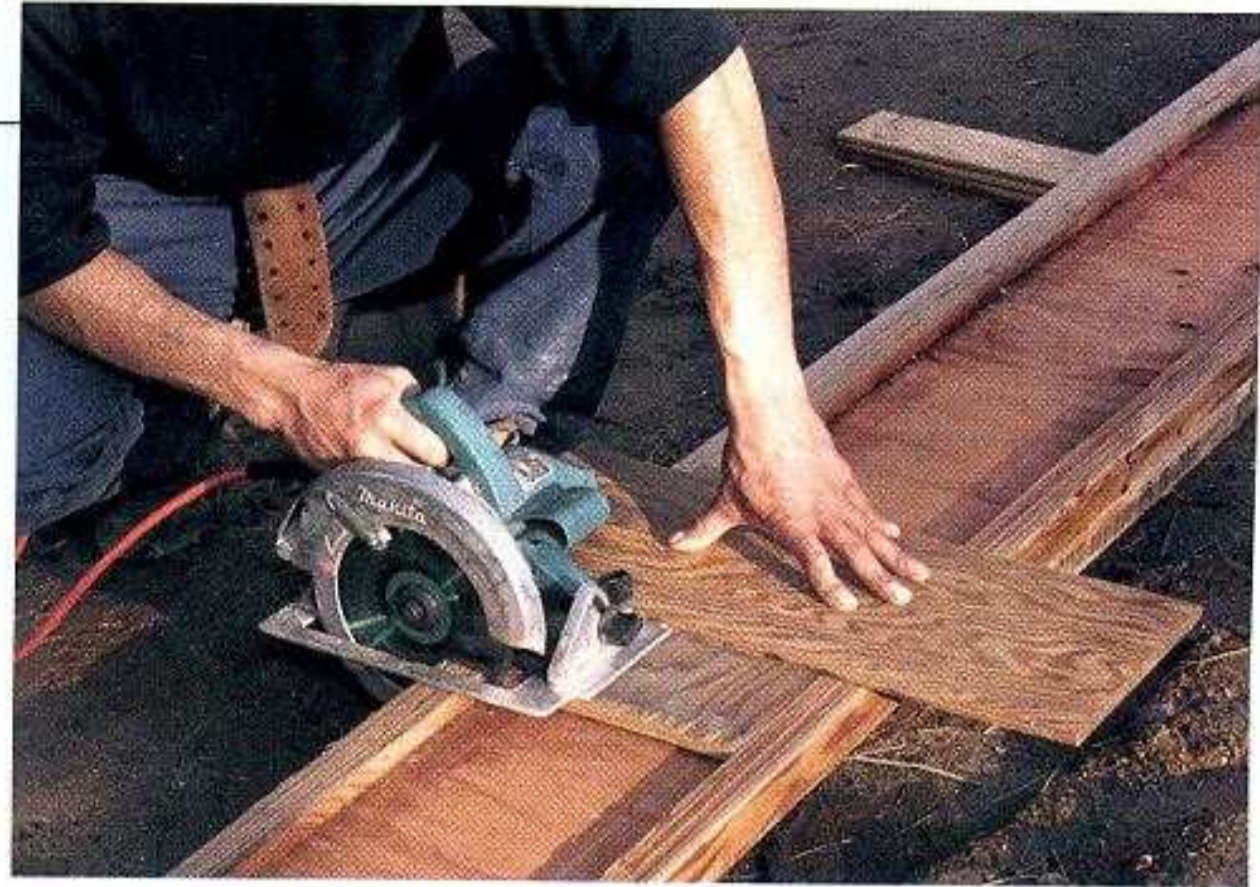
CUT I-JOISTS WITH A GUIDE. Scrap sheathing that is nailed or screwed together creates an effective guide for cutting I-joists. [Photo by Roe A. Osborn, courtesy Fine
