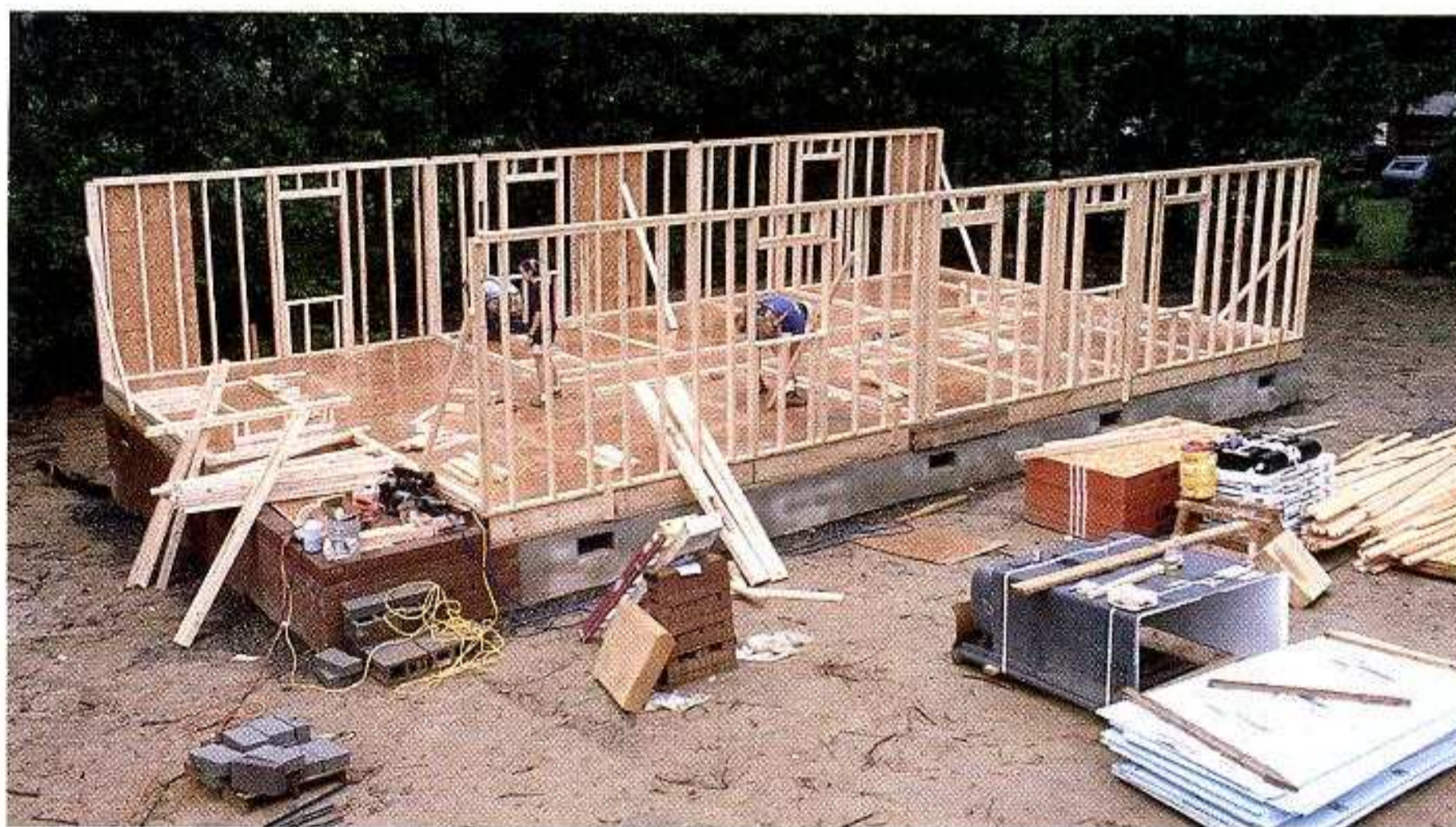
DIAGONAL BRACES ARE IMPORTANT. Both exterior through walls are up; diagonal braces hold them securely while the other walls are raised. Use these temporary braces liberally where needed.
