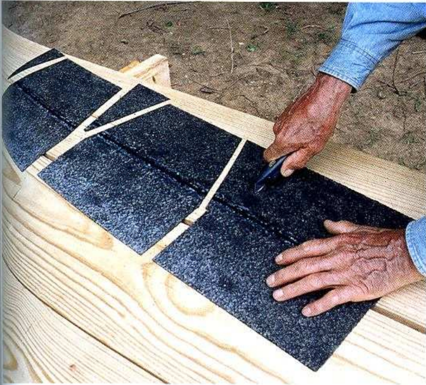
MAKING RIDGE SHINGLES. Cutting a regular shingle into three pieces with a utility knife is an easy way to make these smaller shingles, which will cap the ridge.
