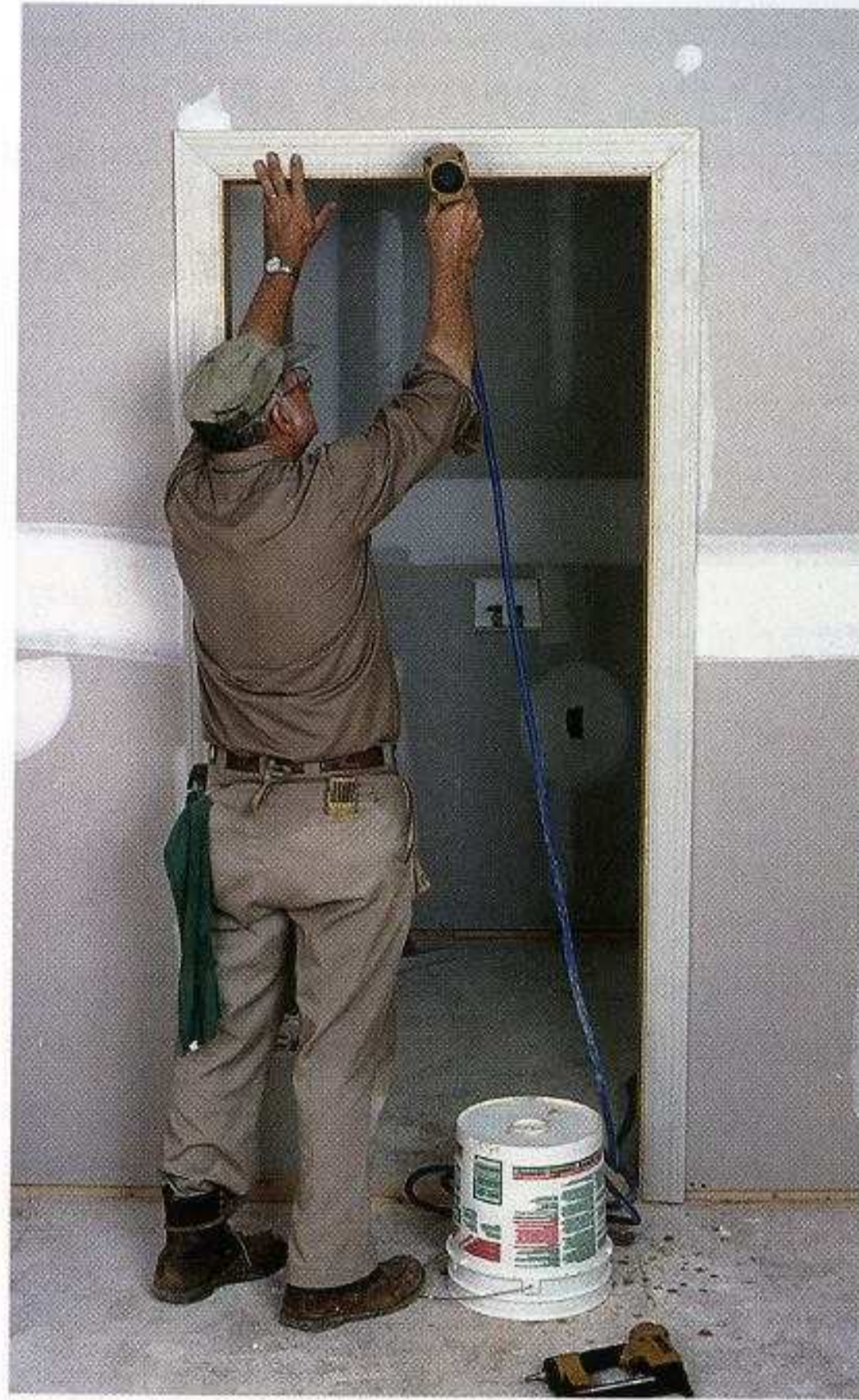
LEAVE A REVEAL. Install the casing so its inside edge sits back a uniform distance ( \frac{1}{4} in. or so) from the corner of the jamb. This creates a pleasing reveal.
