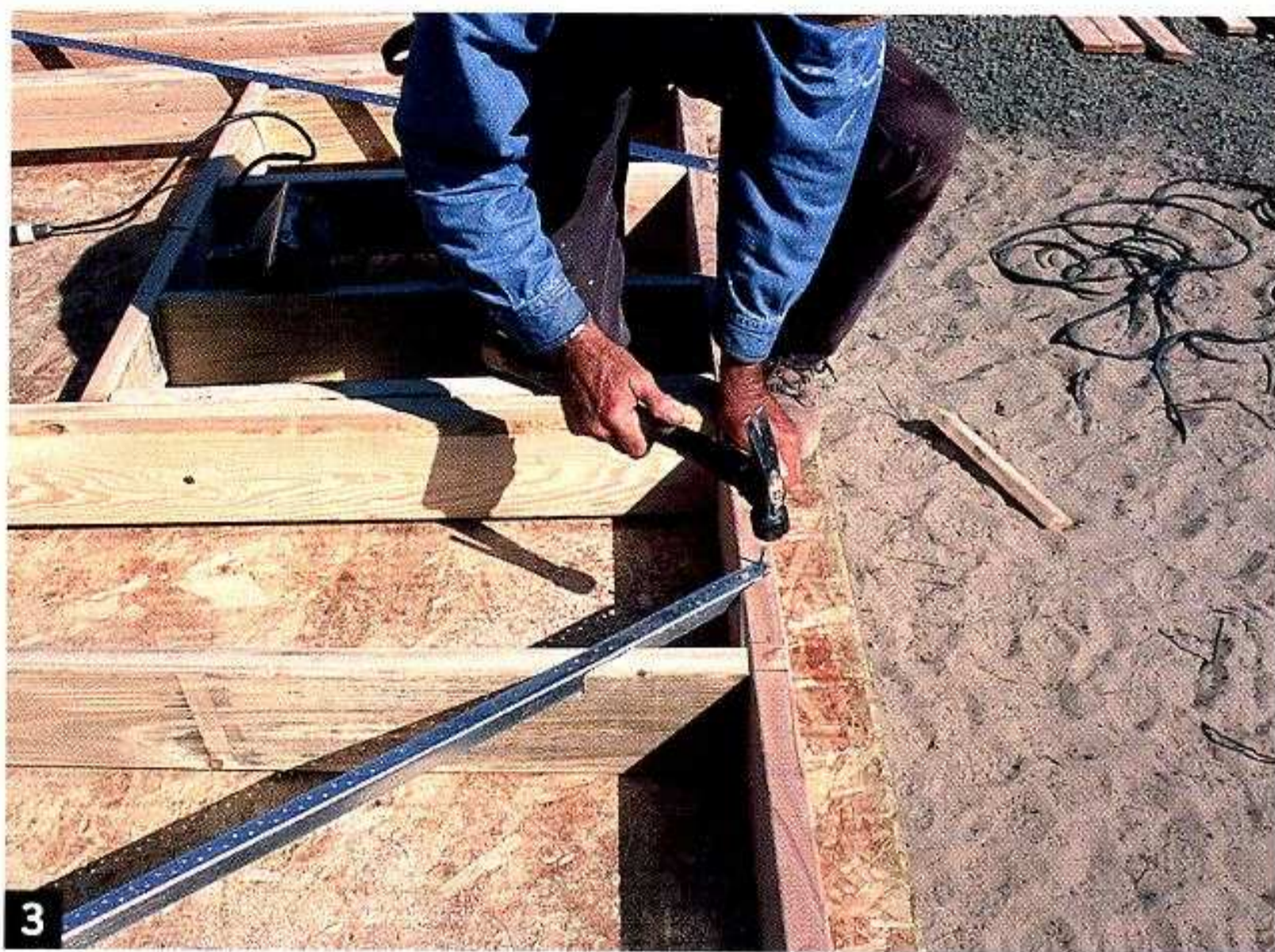
3. Nail off the bottom of the brace. Slip one flange of the brace into the slot and nail it to the bottom plate with three 8d nails. Drive one more 8d nail through the brace and into the first stud. At the double top plate, start an 8d nail alongside the brace and bend the nail over to hold the brace in place as the wall is raised.
