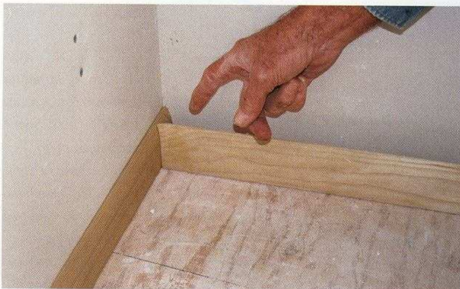
INSIDE BASEBOARD CORNERS ARE COPED. The coped cut fits the profile of the trim piece that runs into the corner. [Photo © The Taunton Press, Inc.]
