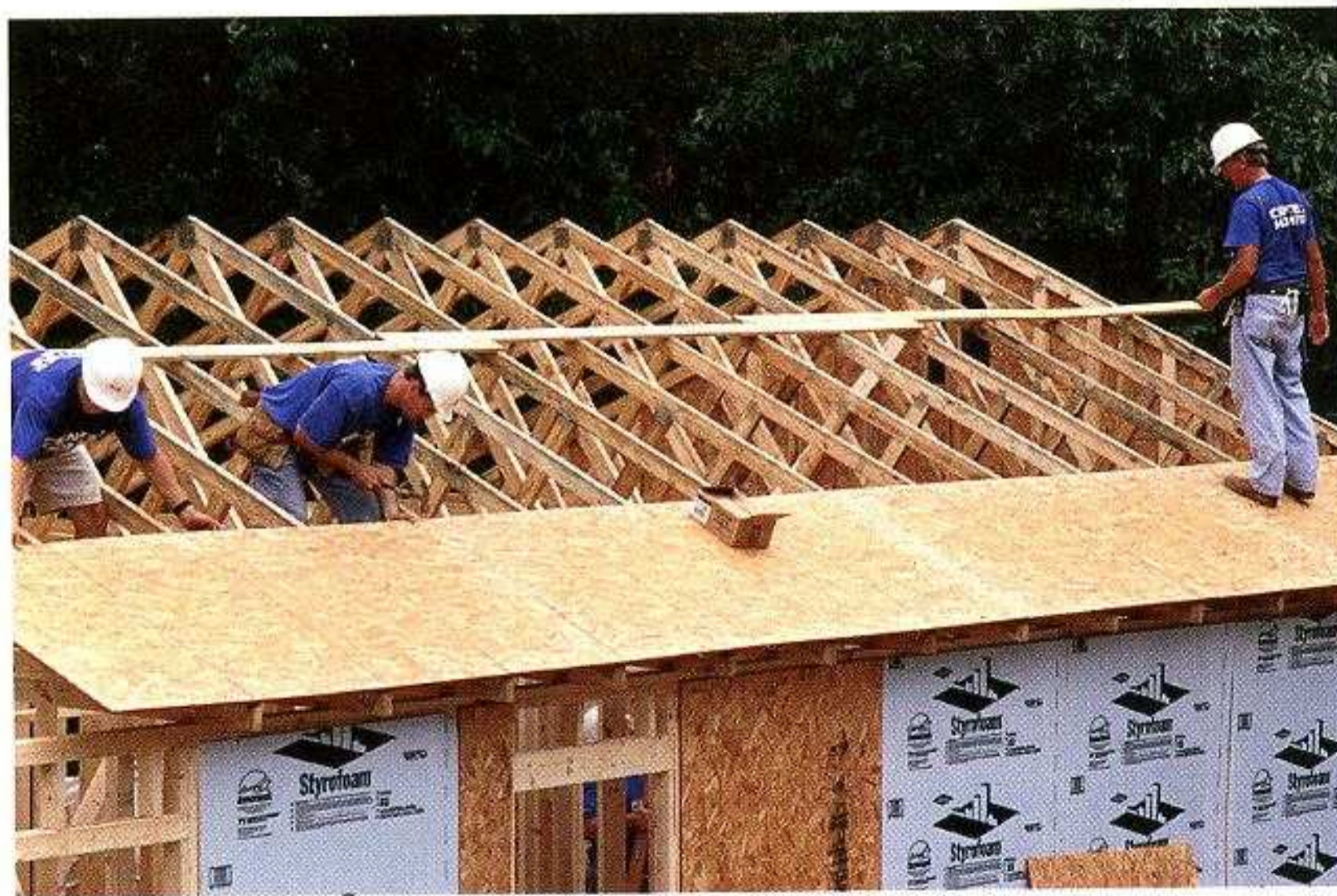
SHEATHING WORK BEGINS. Position the first row of sheathing with the top edge against a snapped reference line.
