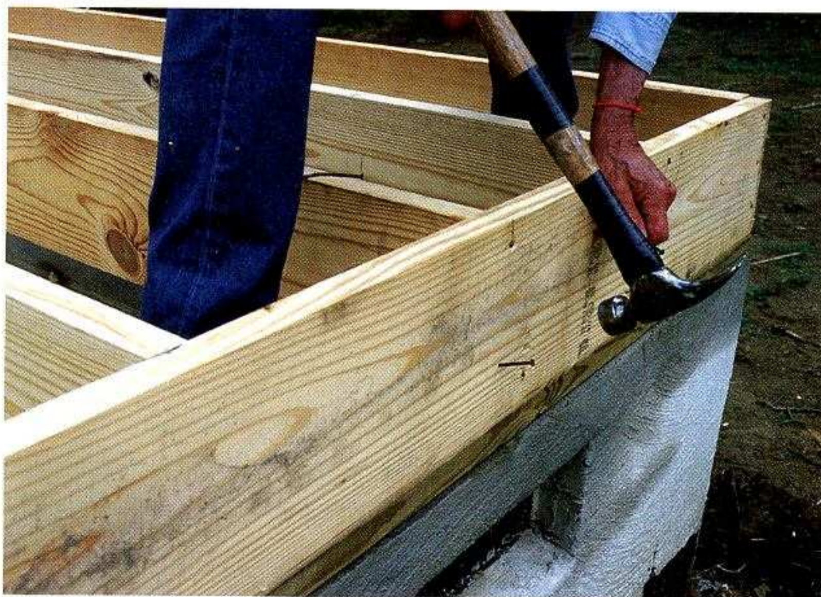
NAIL OFF 2x JOISTS. To install 2x joists, drive a pair of 16d nails through the rim joist into the end of the joist. Then drive a toenail through each side of the joist into the sill.
