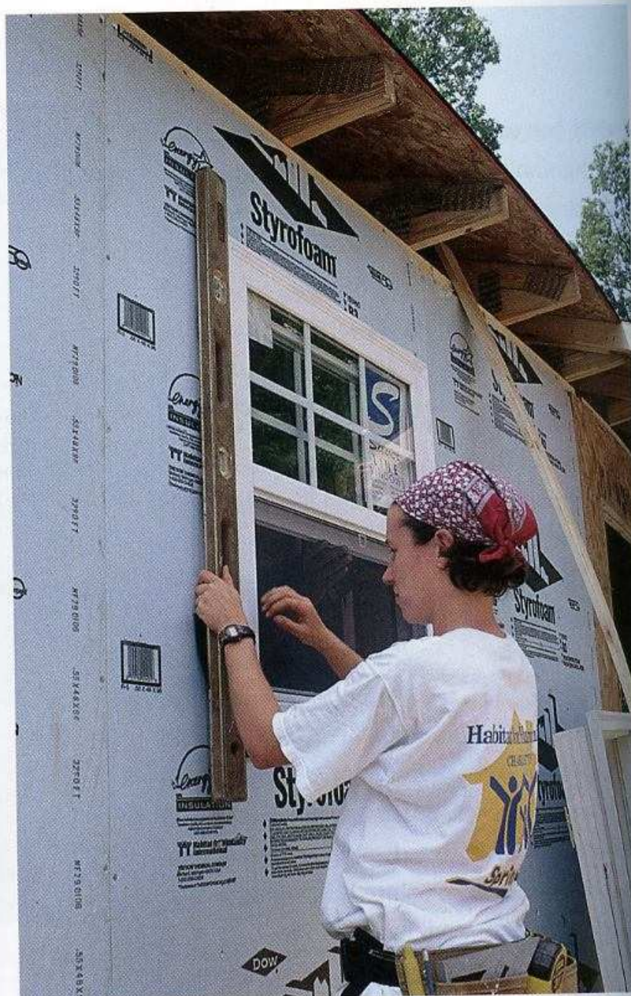
PLUMB THE FRAME WITH A LEVEL. Before nailing the flange to the wall, fine-tune the window's position so the side of the frame is plumb.
