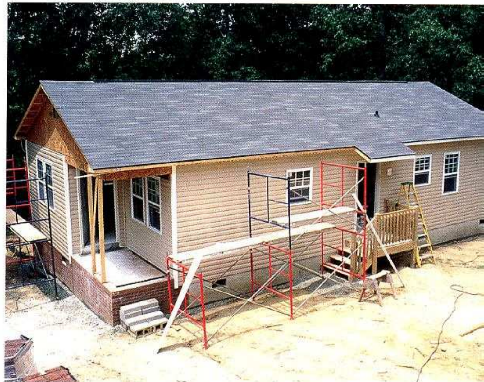
READY FOR RAIN. Finishing the roof is a big step forward. High-quality roof shingles should last 25 years or more and require little or no maintenance.
