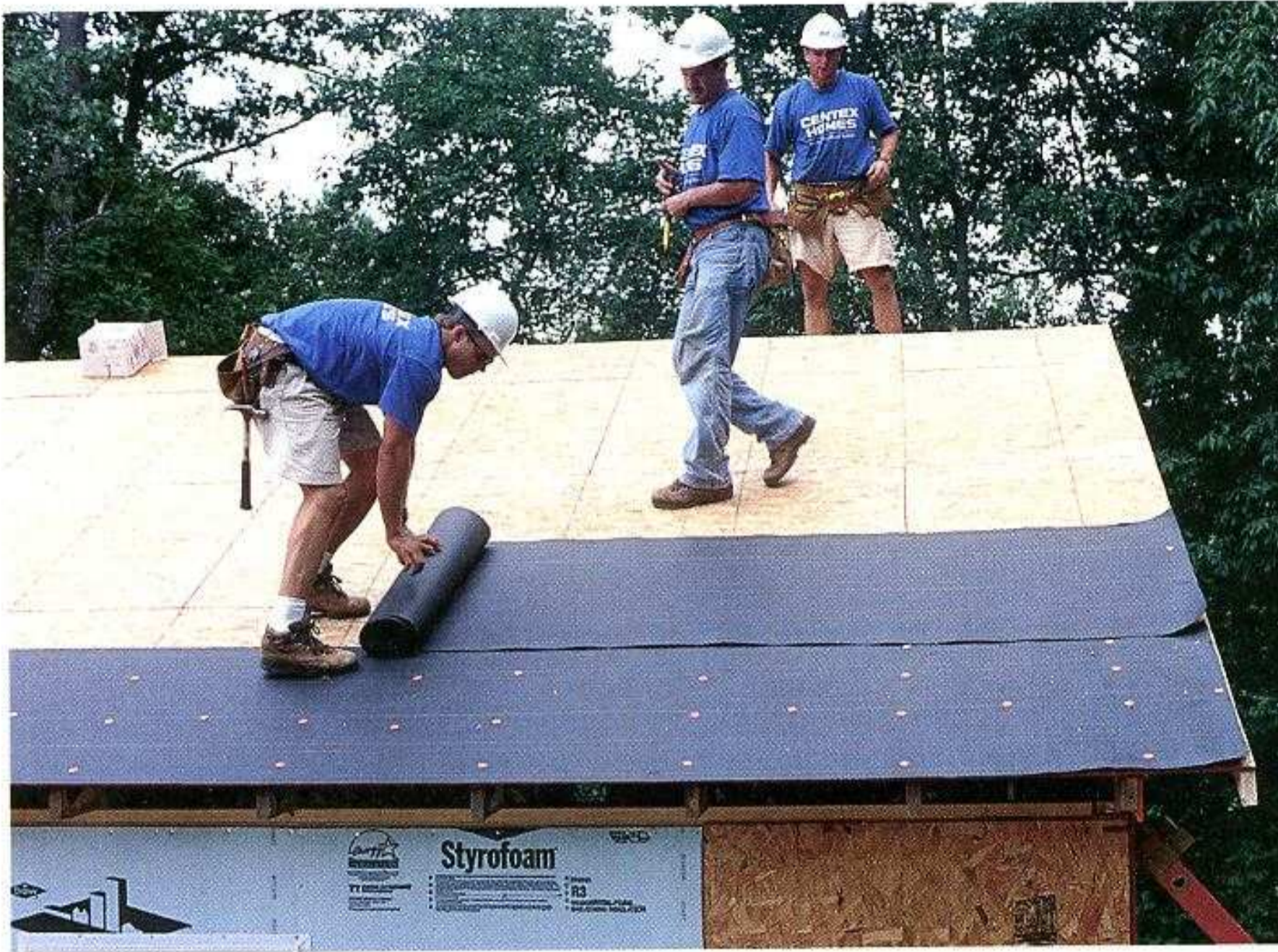
ASPHALT PAPER IS THE FIRST LAYER OF PROTECTION. Known as builder's felt, this waterproof paper is applied over roof sheathing. Overlap each course by at least 4 in.
